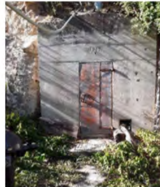
Photo 1. Government Springs, view of entrance to bunker that houses the spring box, September 2019
