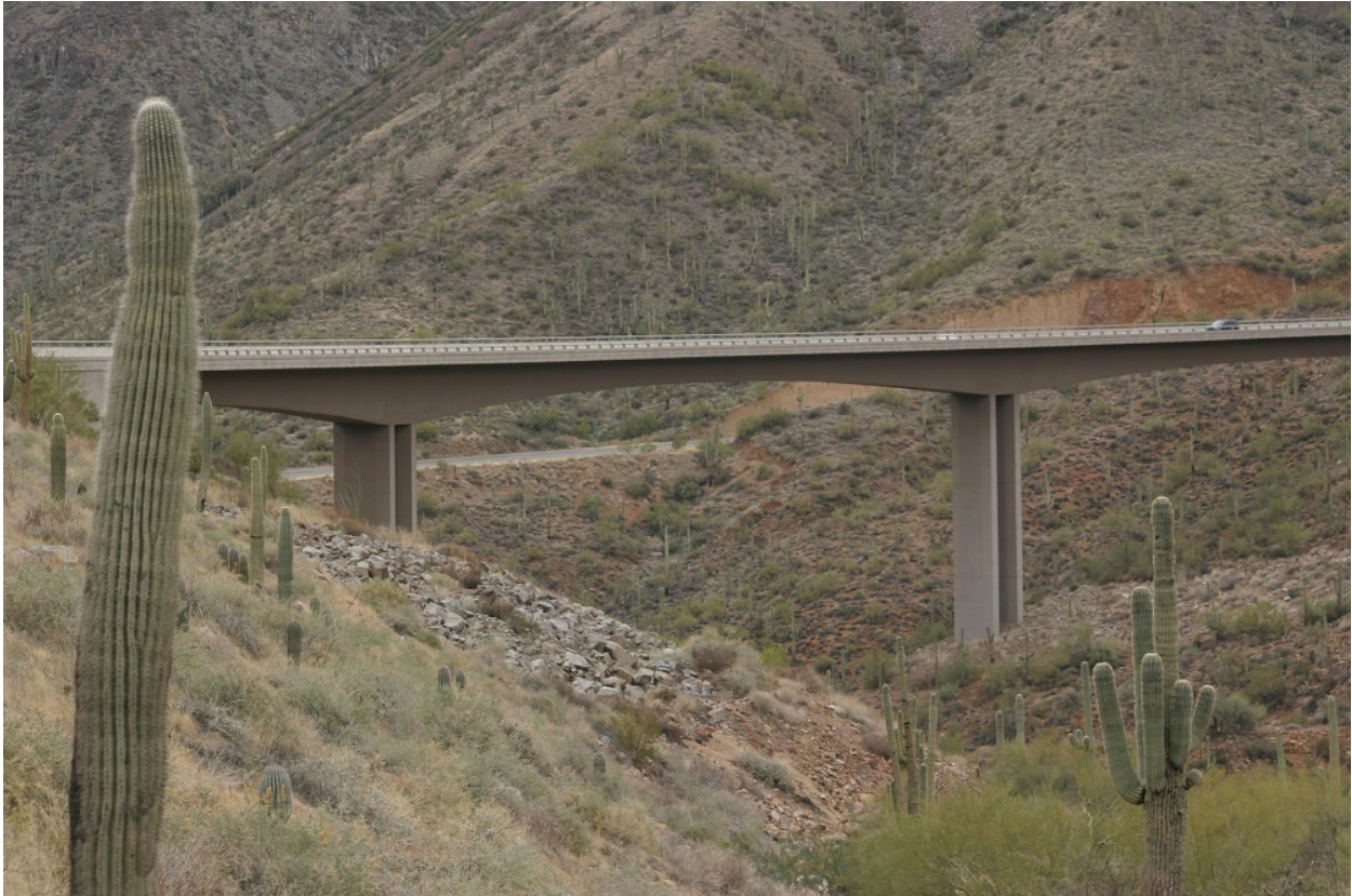
Figure 3.5 With larger dimensions, long spans between bridge supports can have less of an impact on sensitive wildlife corridors while allowing traffic to move overhead.
