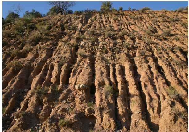
Figure 4.12 Eroding slopes stand out as an eyesore and continuously add silt to highway ditches.
