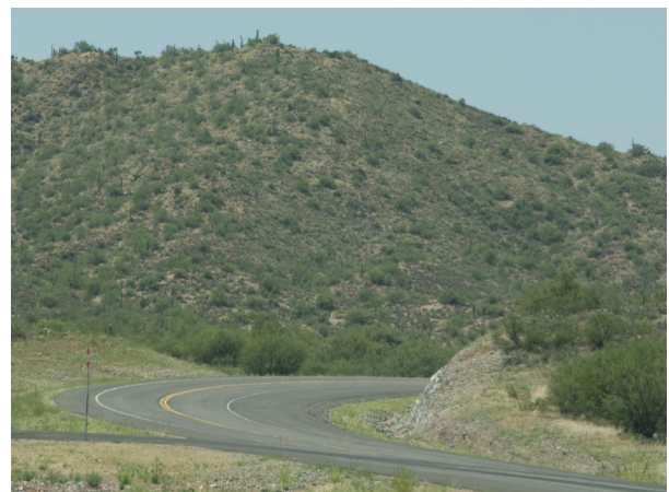
Figure 4.18 Warping so that the cut face is not parallel to the roadway.
