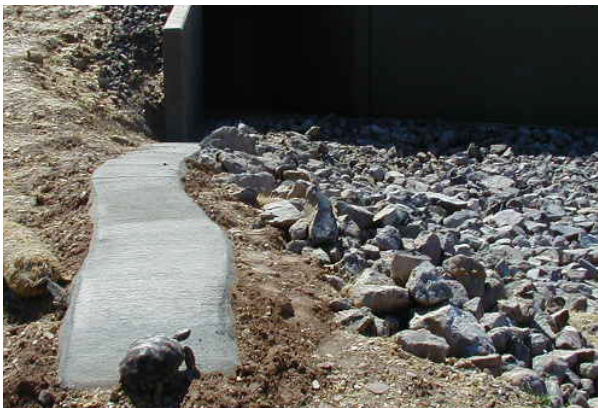
Figure 3.14 Successful tortoise underpass on US 60.
