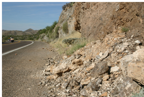
Figure 11.6 Cleaning of ditches below slopes includes cleaning the occasional build-up of rock fall.
