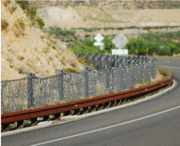
Figure 4.27 Fence at edge of ditch area to stop rock fall from entering roadway.
