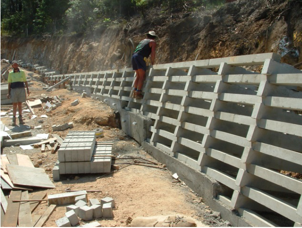
Figure 4.32 Crib walls can be open or closed, made of wood or concrete.
