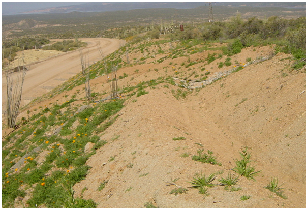
Figure 6.5 Crown ditch installed at the top of slopes to divert sheet flow.
