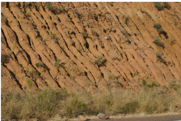
Figure 4.9 Long steep slopes are prone to erosion damage.
