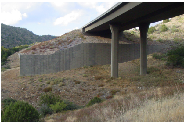
Figure 6.12 Protection from erosion at edge of bridge abutments.
